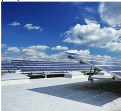
Solar Panels in a rooftop
