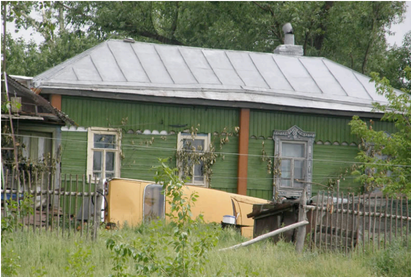
Figure 115. Damage from tornado in Zaria Svobodi, Russia, 2009-06-13, courtesy Kyle and Svet Keeton .
